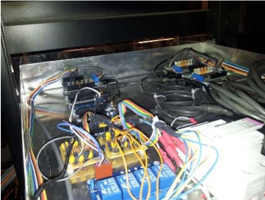
FIG. 2. A close up of the Arduino inside of the control box.
